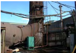
Chimney Bag Filter Exit
