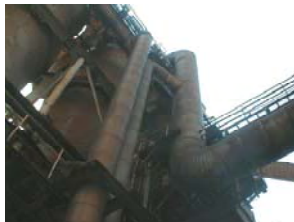
Blast furnace Exit
